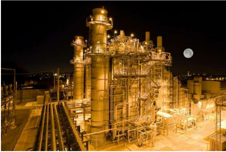
MONITORING & AUTOMATION OF INDUSTRIAL PLANTS
