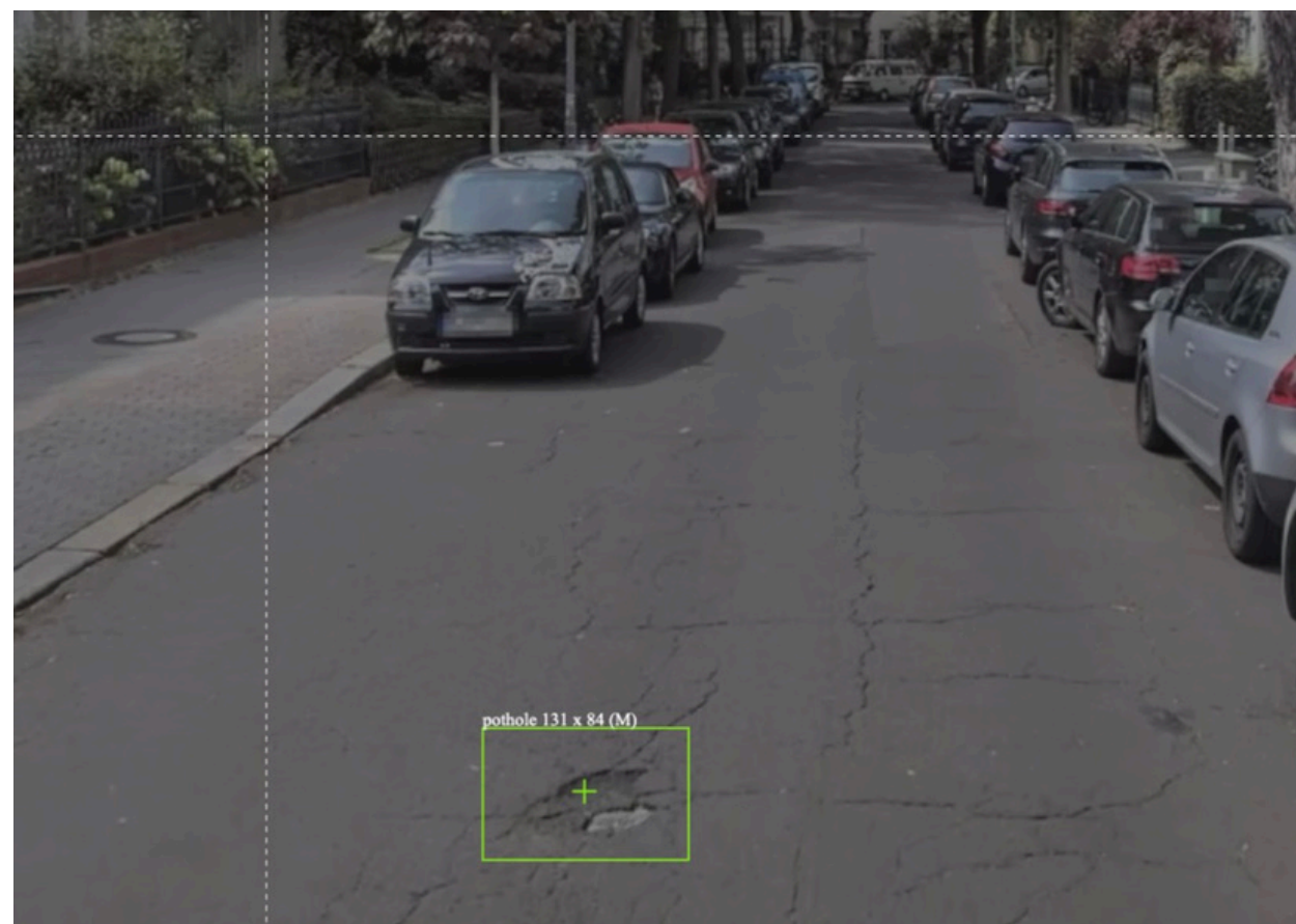
POTHOLE, STREET CONDITIONS
